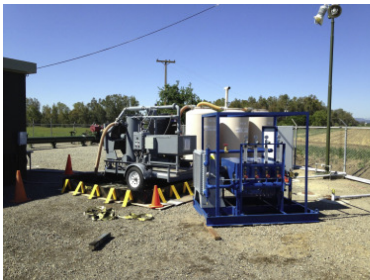
Figure 11.6. Soil vapor extraction and air sparging systems.
